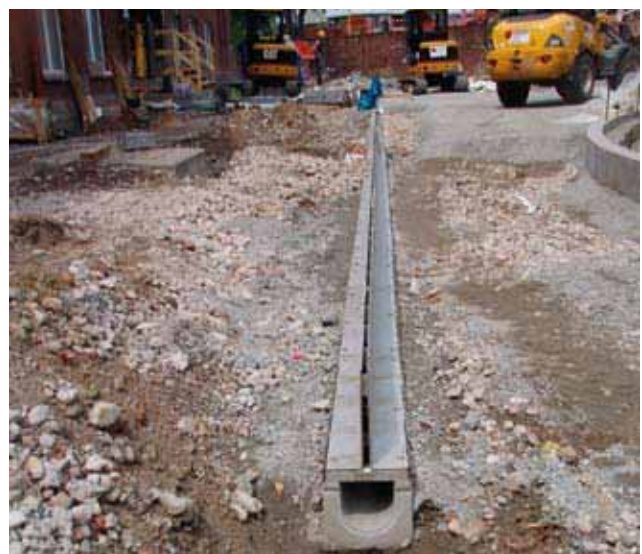
Installation of the solid Design slotted channel with grating made from 4 mm thick stainless steel and 280 mm neck height.
